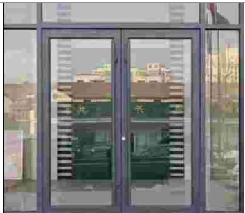
2 - Aluminium Door & Double Glazed Glass Color to Match: Benjamin Moore Black Ink 2127-20 Glass: Clear
